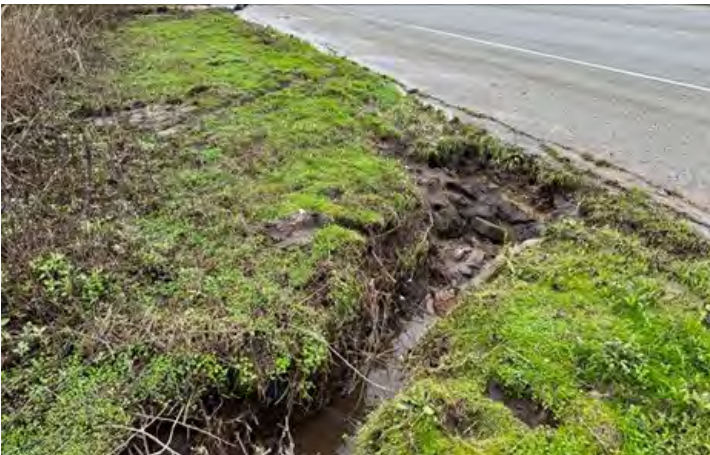
This diverter saved the driveway entrance.
