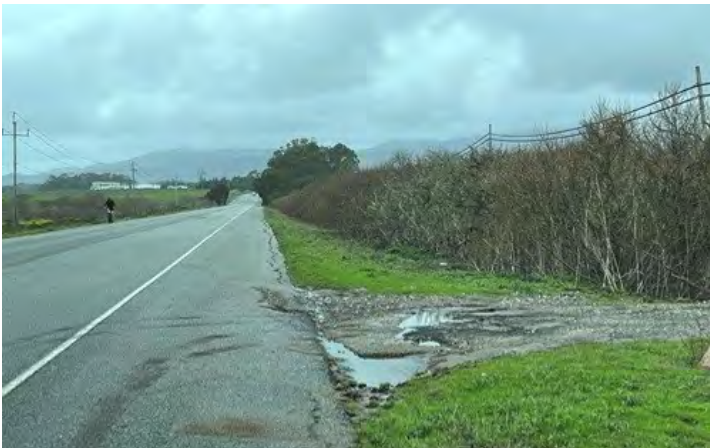
The entrance was in a rough shape!
