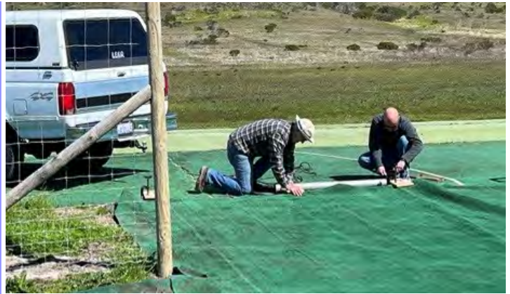
Dave Santana and Roberto Ourique on the job. Brian Chan was taking photos (and nailing the astroturf down!)
